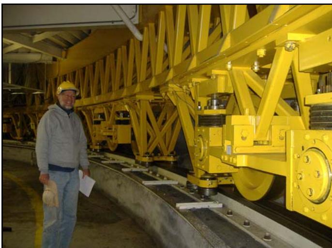
The entire Subaru building rotates on dozens of massive wheels. Russ gives perspective to their size.
